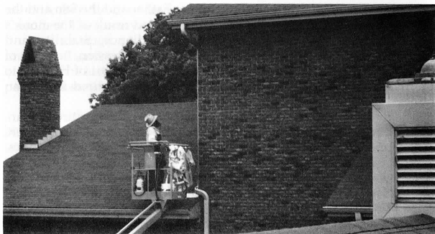
Father Francis among the roof tops! We do our own repair work.
