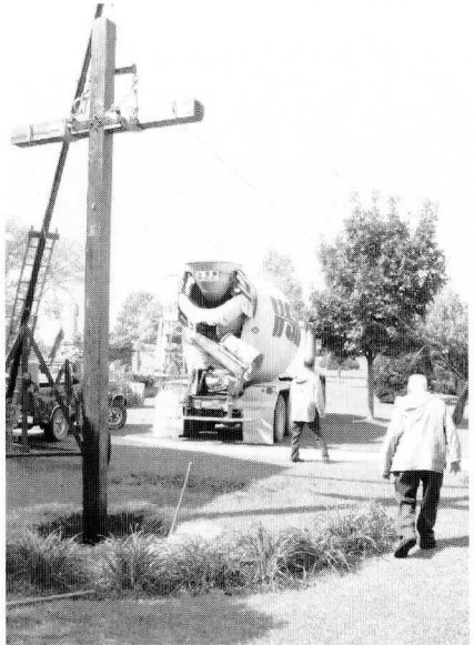
The concrete is then poured into the hole which is approximately five feet deep and five feet across.
